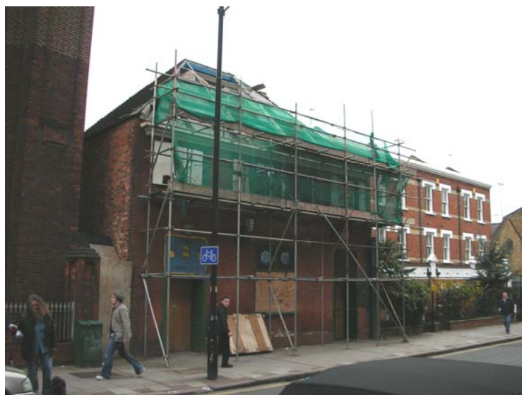
Nos 39-40 Cornwall Road are in poor condition and require immediate attention.
